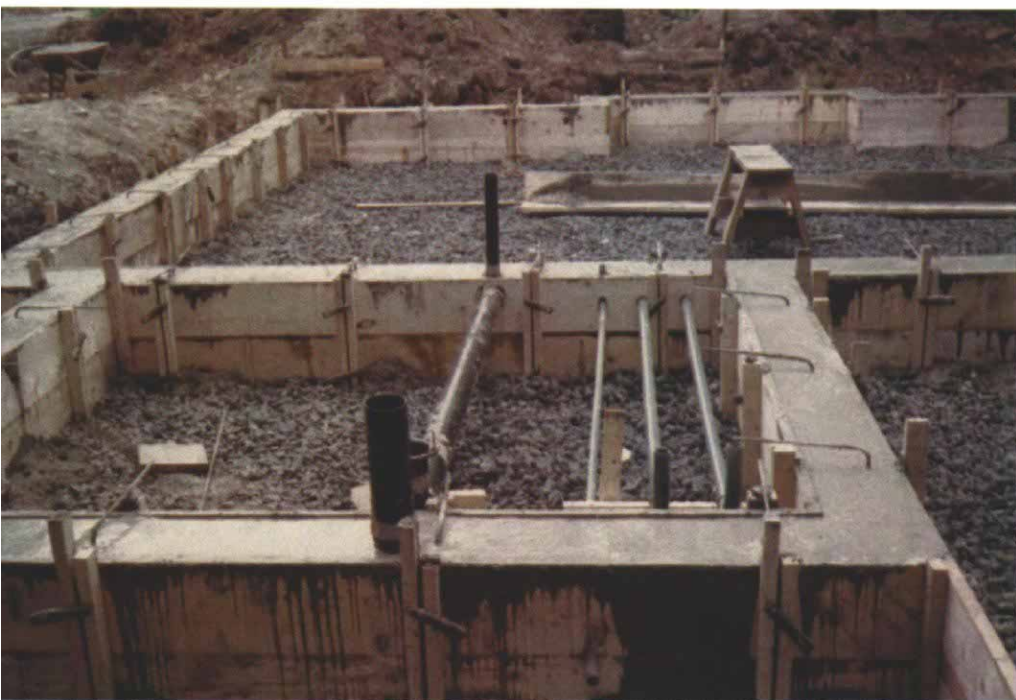
The top of the modified grade beam was screeded off with a 2x4 and left rough for better bonding to the slab. The strongbacks extend above the 2x12s in order to serve later as supports for the 2x6 slab form. While the concrete cured, the right-angle rebar, which would tie the slab to the beam, was held at the proper angle by stone shims on top of the 2x4 strongbacks.
