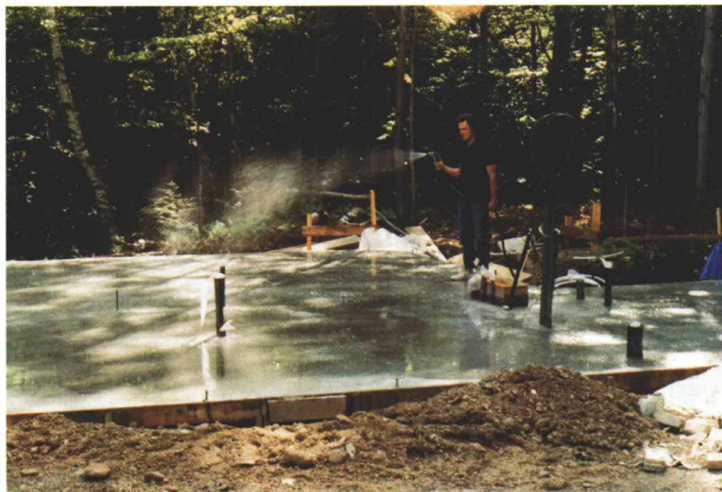
In order to keep shrinkage cracking to a minimum, the slab was kept wet for several days after the pour, allowing the concrete to cure evenly.
