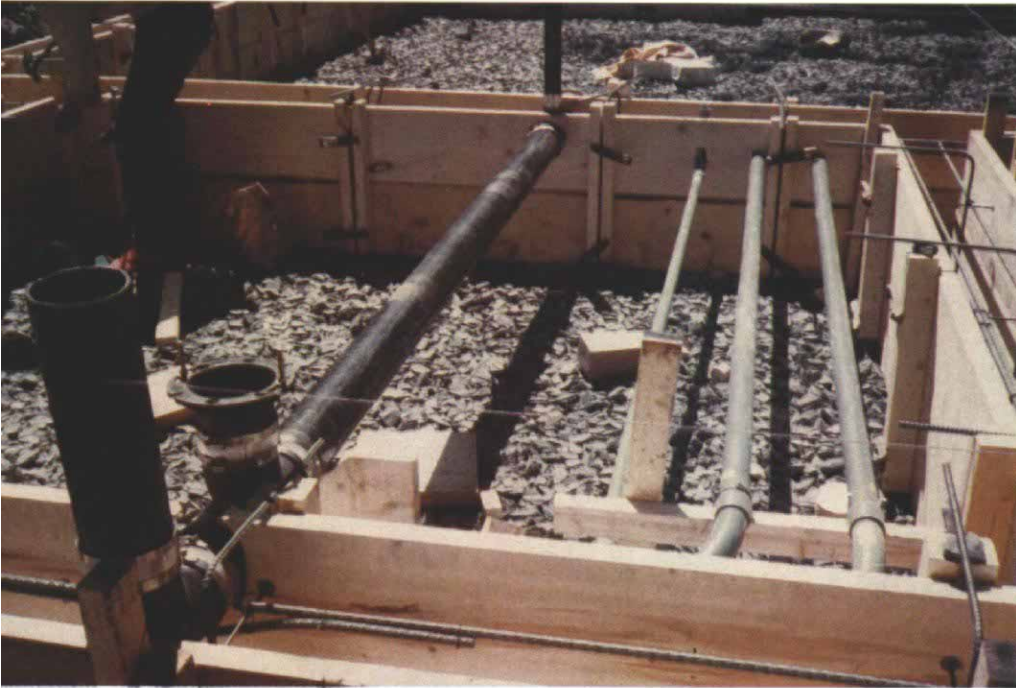
The vent stack, toilet drain, and other waste and supply lines that penetrated the modified grade beam had to be carefully positioned before the pour.
